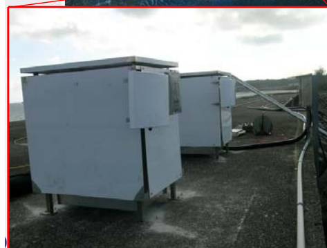
▲ Outdoor IPv6 Smart Sensor Server
